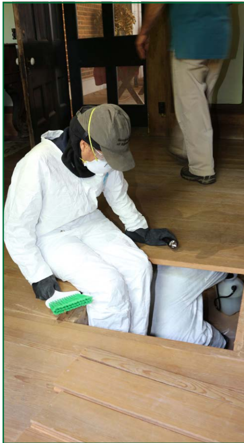
Inspectors access a crawl space beneath the dining room at Valley View through a trap door in the floor.
