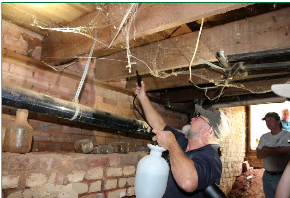
Inspector Carl Schnabel, who previously worked as a pest control professional, leads a demonstration on the proper application of Bora-Care in one of the more generous crawl spaces at Valley View.
