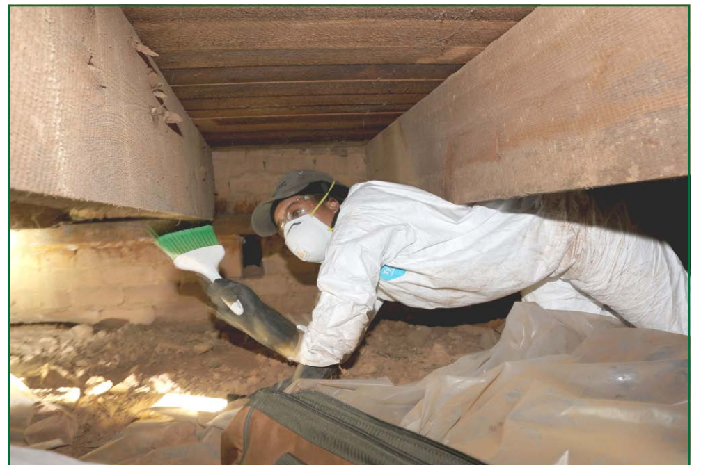
Inspector Kiara Knight brushes away powder post beetle frass and cobwebs from the joists in a crawl space prior to applying the Bora-Care treatment. (Photos by Amy Carter/GDA)
